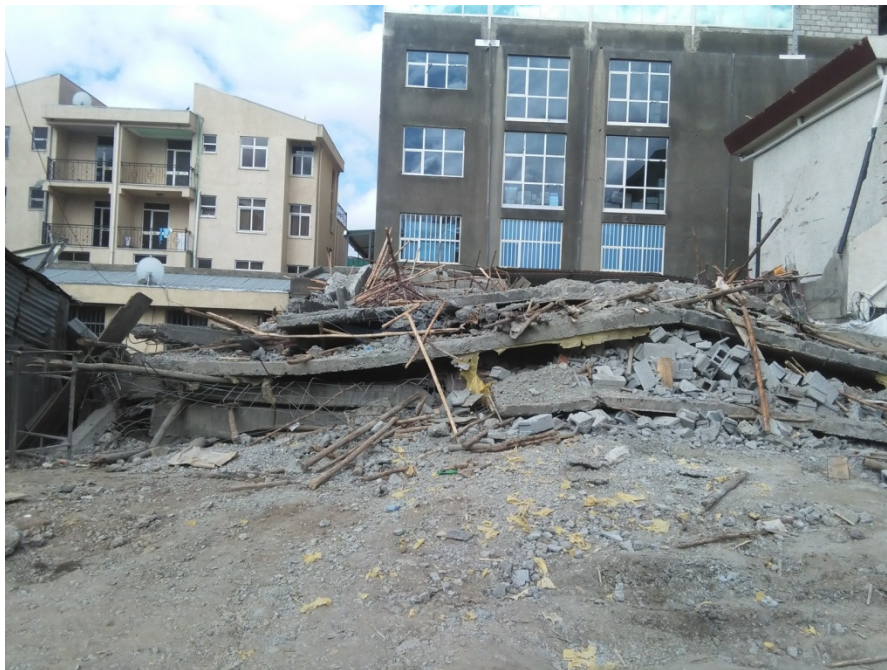
Figure 6.3 Bole sub city Wereda 10 three storey building that collapsed on 14 February, 2017
