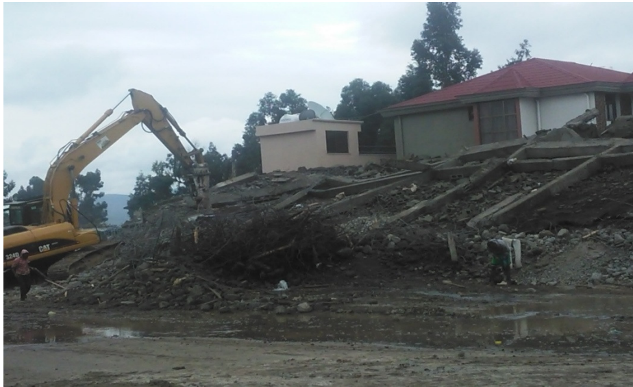
Figure 6.2 Bole sub city Wereda 10 five storey building that collapsed on April 27, 2016
